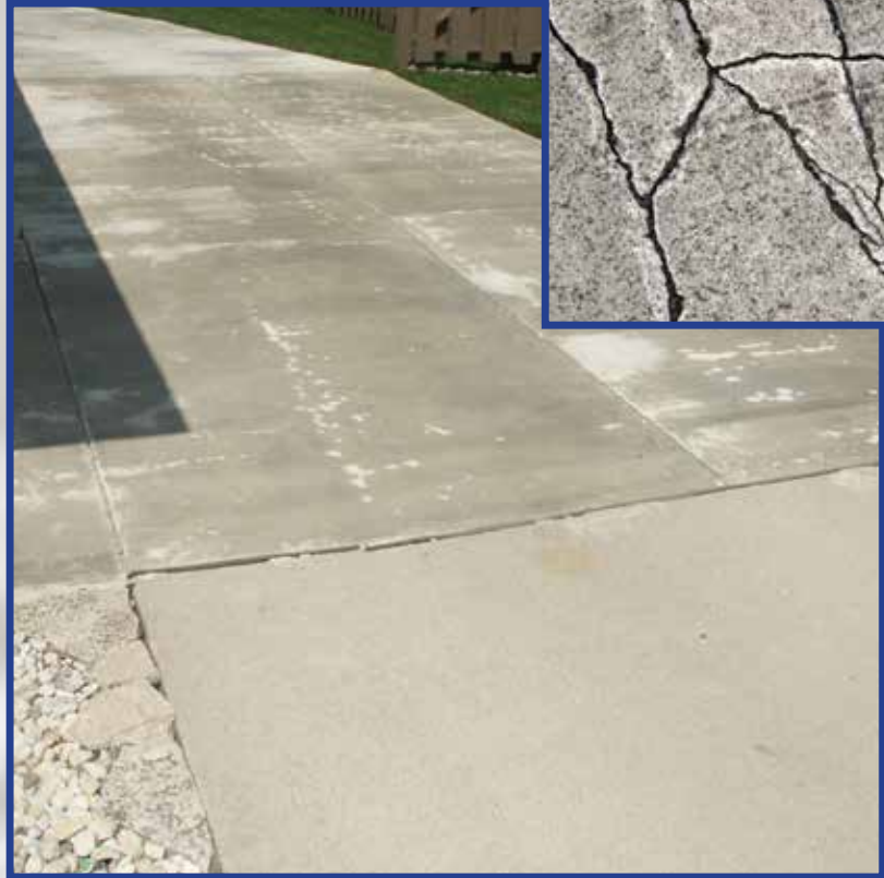
This is an example of concrete that would be at risk of damage to increased freeze/thaw cycles.
